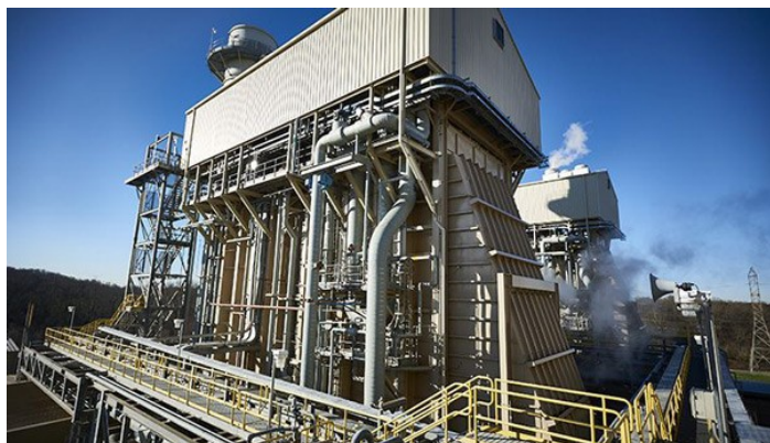
Buck combined cycle plant
